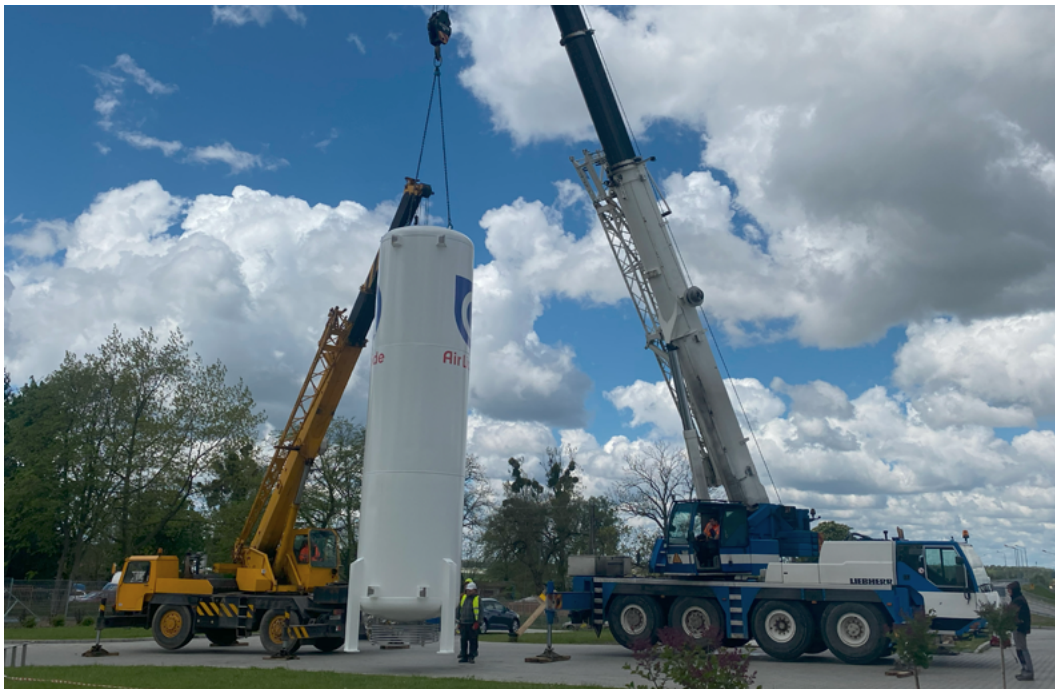
Photo 11. Installation of a liquid nitrogen tank at the manufacturing facility in Załuski.
