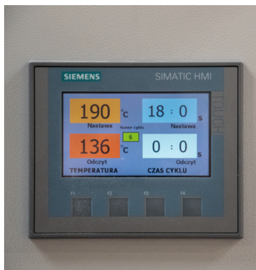
Photo 7. Siemens Simatic HMI control panel integrated into the production furnace.
